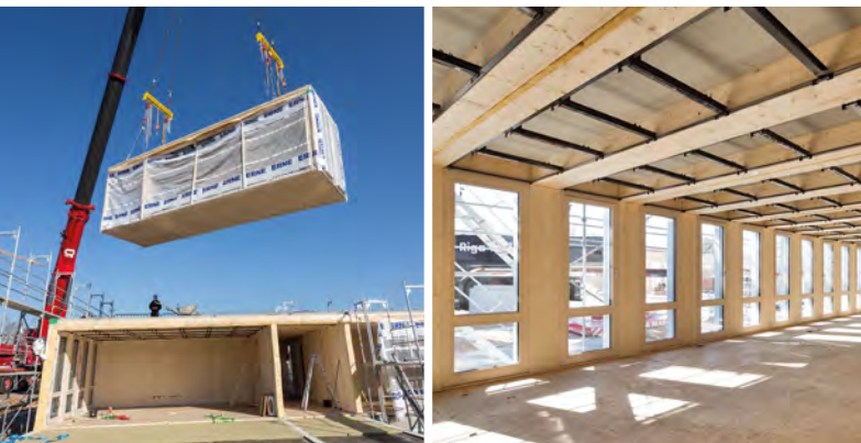
Built by ERNE AG Holzbau based in Aargau, Switzerland, Photograph: Thomas Koculak
